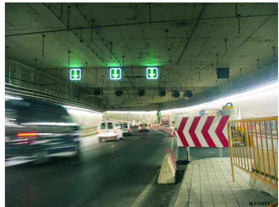
FOGTEC system in M 30 Tunnels
