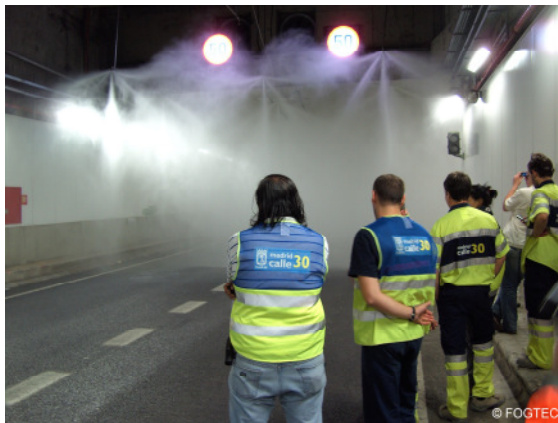
Spray test in M 30 Tunnels
